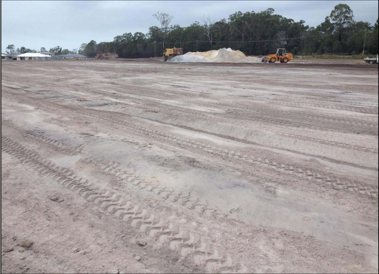
Picture 2: View of the Stripping Operations Prior to the Placement of Fill
